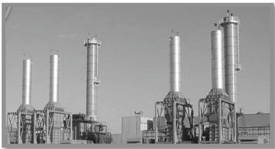
Gas-Fired Turbine Peaker Plant
