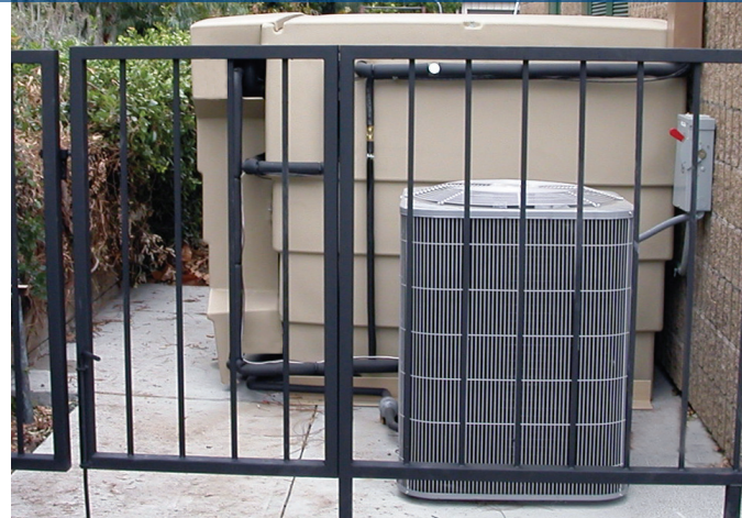
Ice Bear 50™ Distributed Energy Storage System Installation at Anaheim Firehouse No. 8
