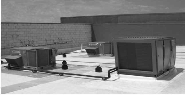
Figure 3 UTSS (right) connected to standard rooftop unit (left). Installation photo.
