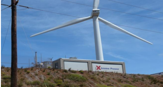
Xtreme Power KWP 1
